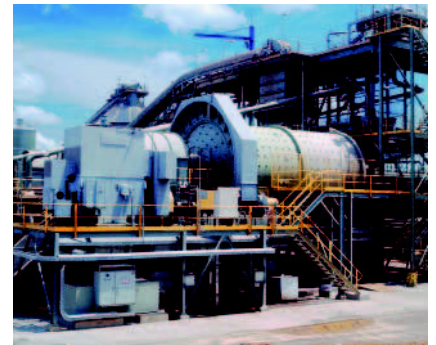
Bearing arrangements in comminution and processing plant
